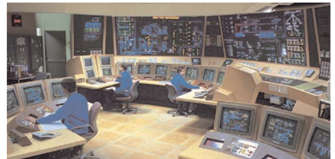
A computerized screen-based control room designed to maximize operator efficiency. Chooz B1, France (N4, 1,500 MWe).
