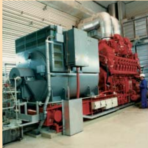
Isar 2, Germany (Konvoi, 1,300 MWe) emergency Diesel generator.
